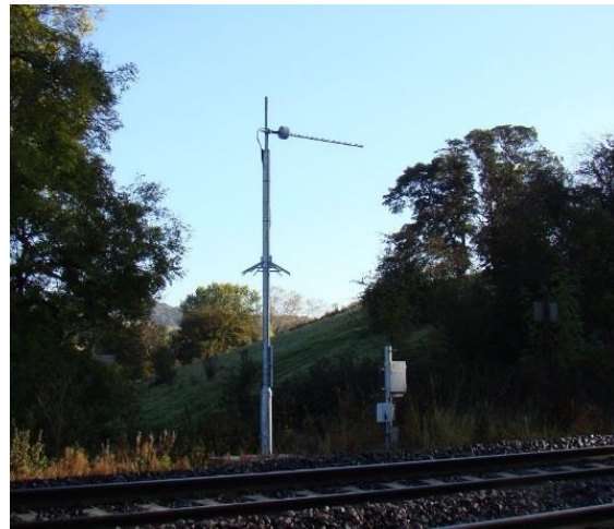
Plate 4.7: A typical pole mounted GSM-R repeater
