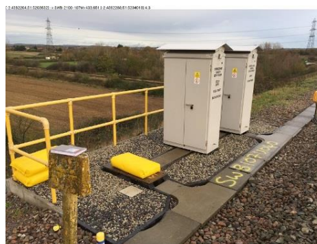
Plate 4.6: An example of LOC Cabinets
